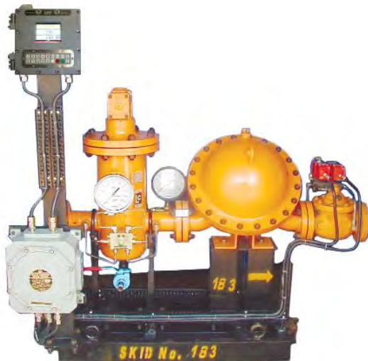
MSA meter skid with Toptech SMP controller
